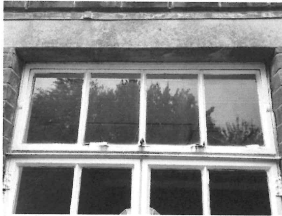
Image 6 Rust jacking to top casement requires attention
