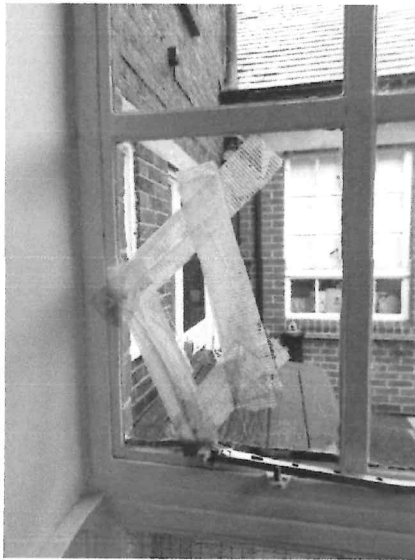
Image 3 Broken panes will need replacing
