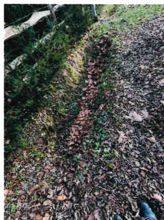
Ditch to front of Old House
