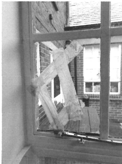
Image 3 Broken panes will need replacing
