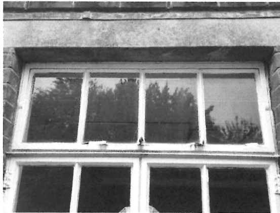
Image 6 Rust jacking to top casement requires attention
